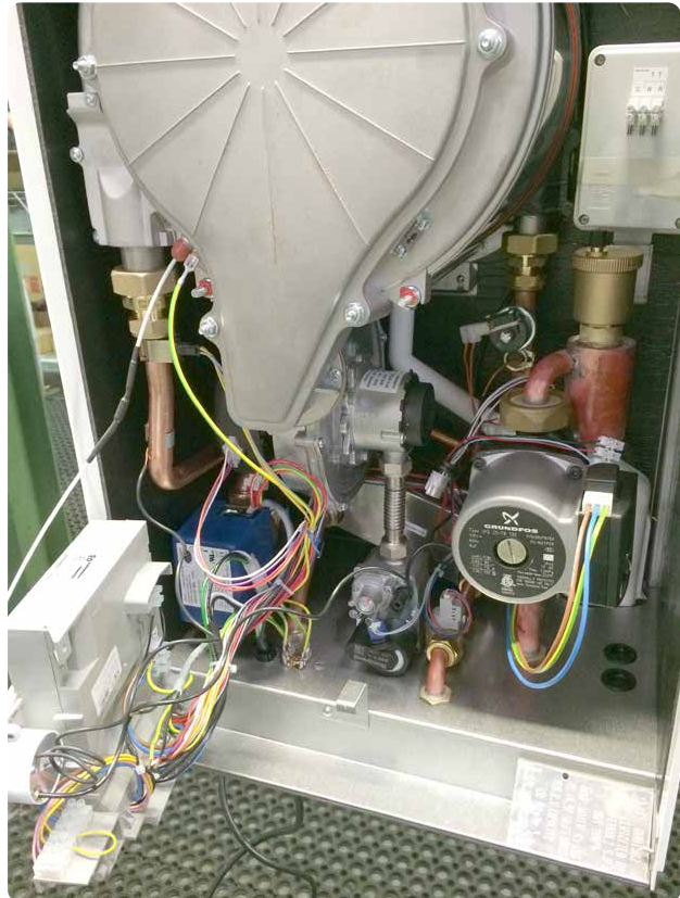
Figure 144 Boiler front panel removed
