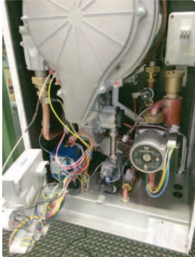
Figure 144 Boiler front panel removed
