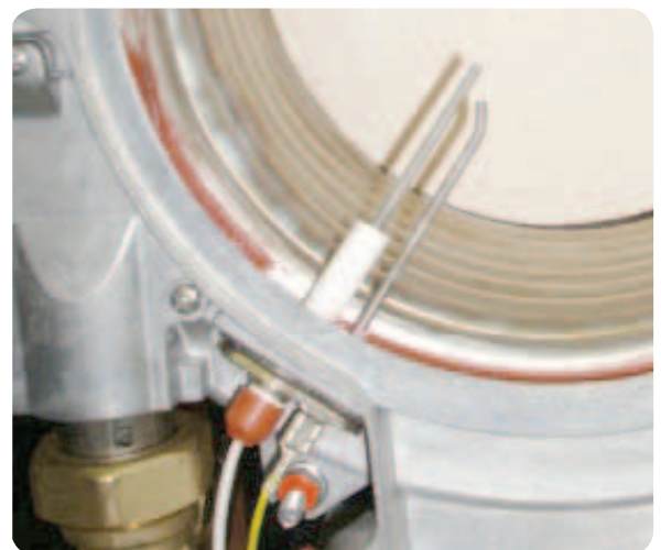
Figure 141 Inspecting ignition electrode
