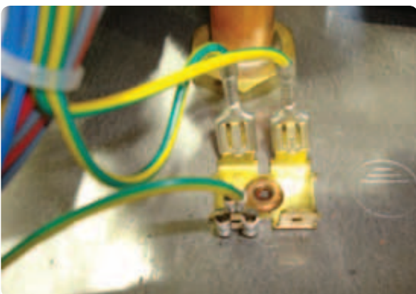
Figure 143 Ignition electrode grounding
